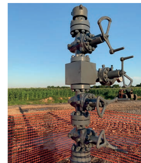
Left: Capped sequestration well. In the industry this set of valves on the well is called the 'Christmas Tree.' This well will be used as a monitoring well once the actual CCS well is operational
